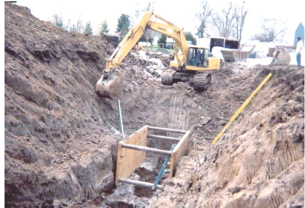
The spoil pile is not at least 2 feet from the edge of the trench and/or retained to prevent it from falling into the trench.
