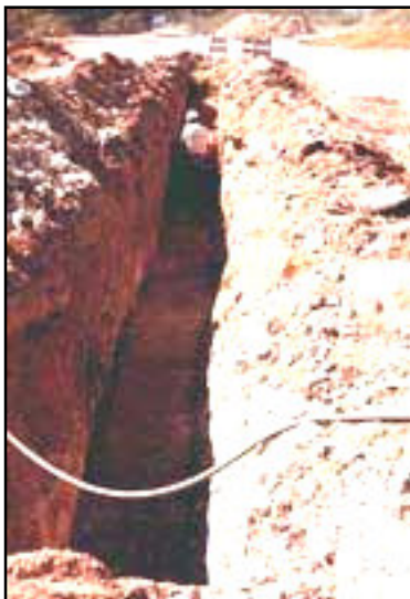
No protective system. No slope or bench. No means of egress.
