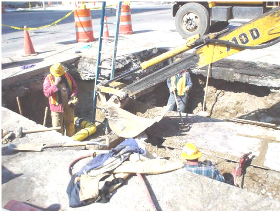
No protective system. Ladder is not angled at 1/4 the working height; it is almost vertical.
