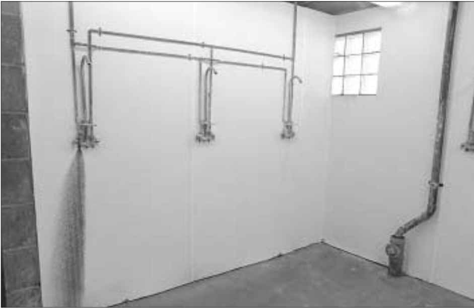
Many migrant worker camps have communal restrooms that all residents must share. In addition to the inconvenience and lack of privacy characteristic of these facilities, substandard plumbing and poor sewage systems cause frequent problems. On busy days, shower drains often become clogged, and sewage water from the toilets reenters through floor drains, flooding the restrooms.
